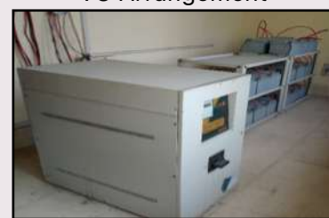
Online Power Backup System
